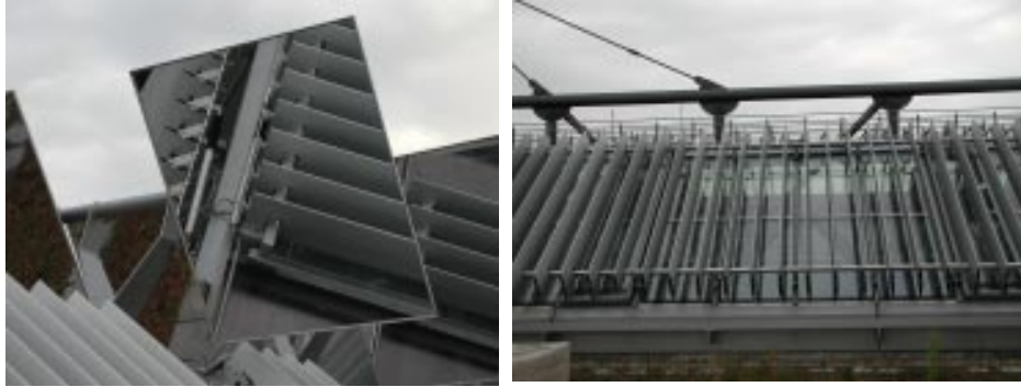
Automated louvers on a skylight system, Technology Museum, Berlin
