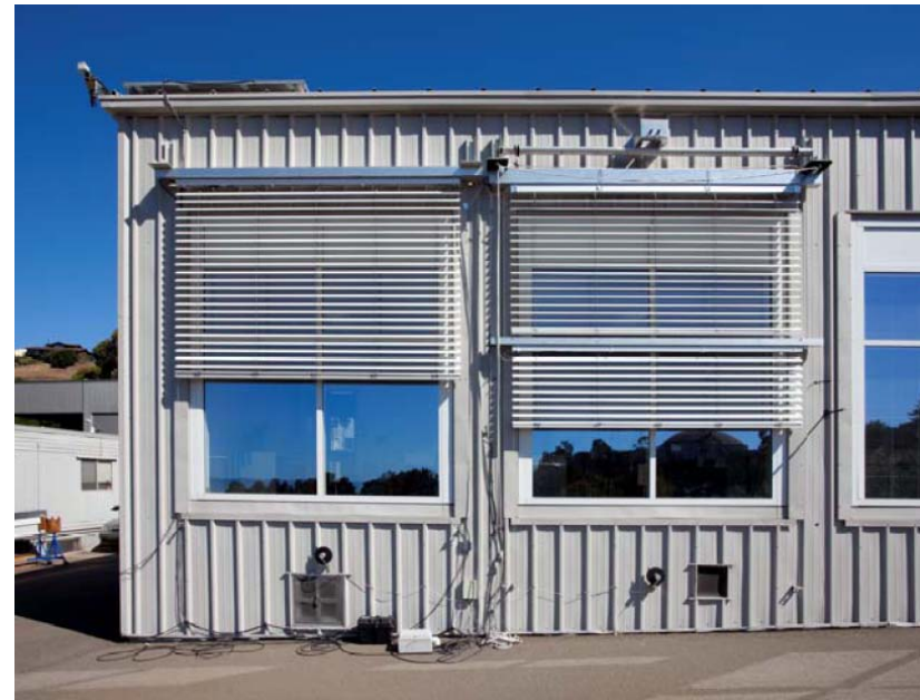
Single zone (left) and dual zone (right) exterior Venetian blinds on the LBNL Windows Testbed Facility. Photo: LBNL.
