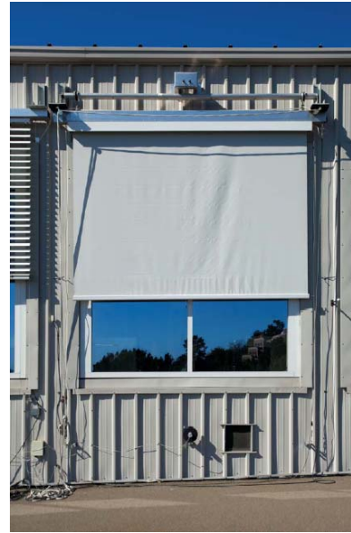
Exterior view of automated exterior roller shade. Photo: LBNL.
