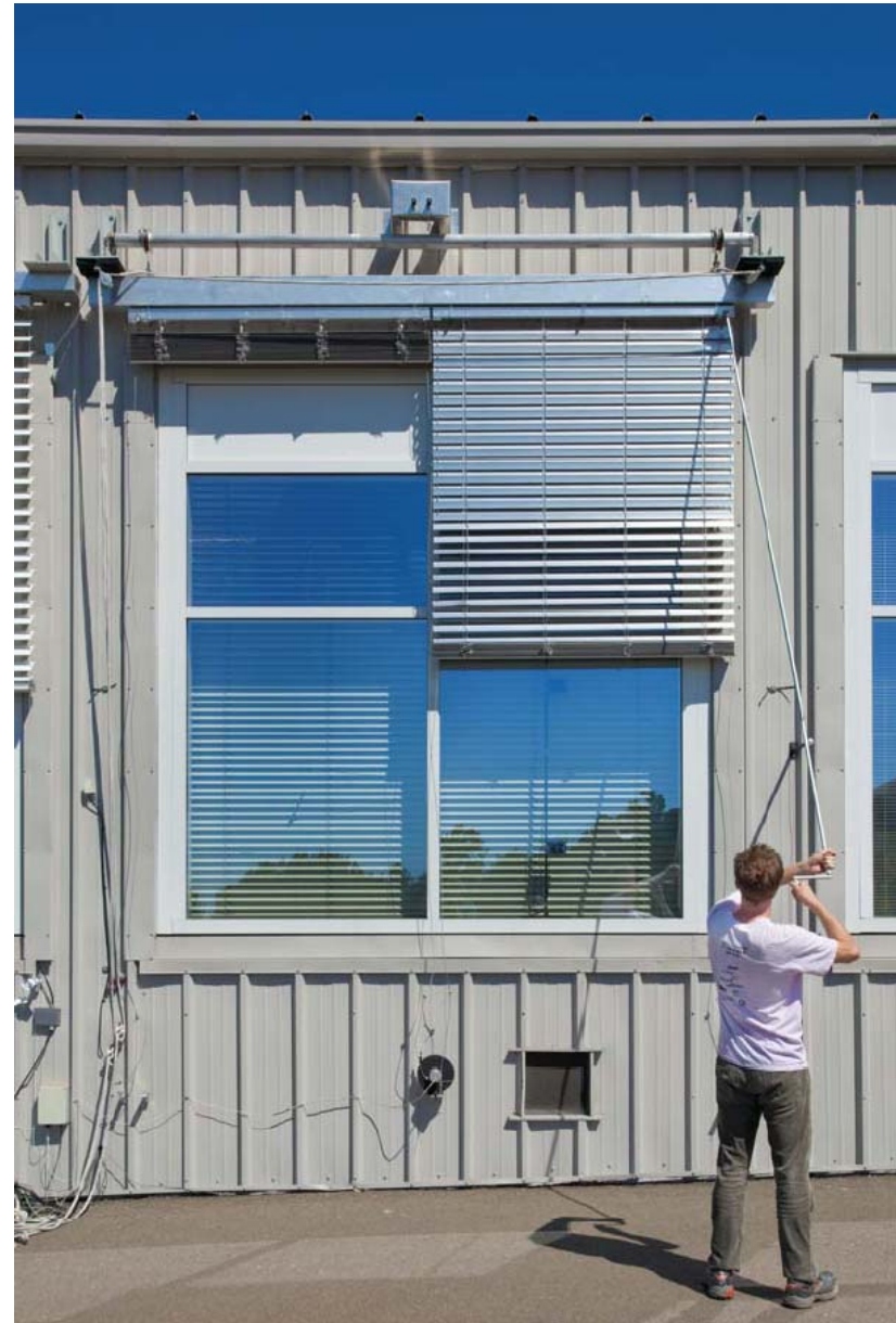
Raising and lowering of an exterior blind using a crank attached to a coupling at the head of the blind. Photo: LBNL.
