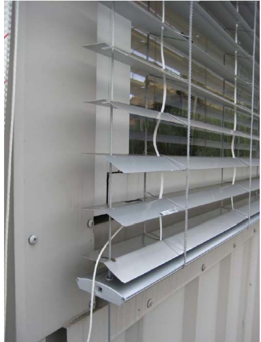
Exterior view of three-zone optical blind. Photos: LBNL.
