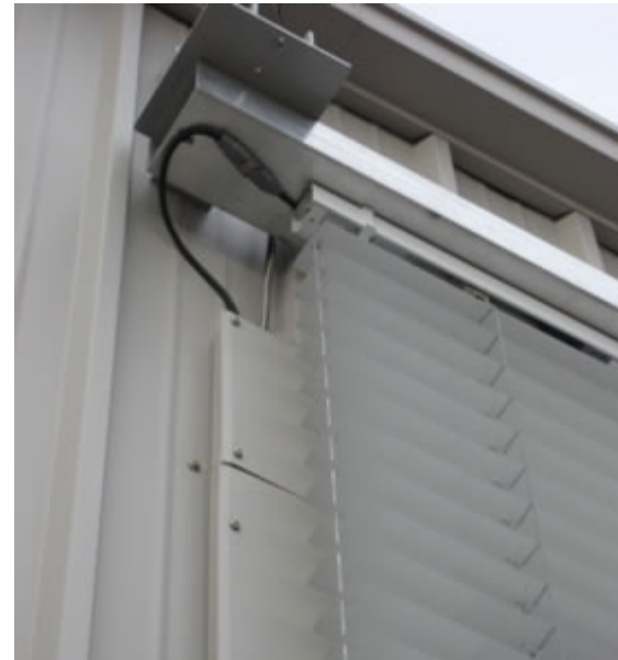
A fixed-speed, runtime-controlled, AC box motor is coupled to a drive shaft assembly and shielded from the weather using a U-channel header (above). Power to the motor is delivered via a pigtail that in this case extended 500 mm from the end of the motor and was terminated with a Hirshmann connector. Ideally the electrical junction is placed inside the building or in a weatherproof junction box. Photo: LBNL.
